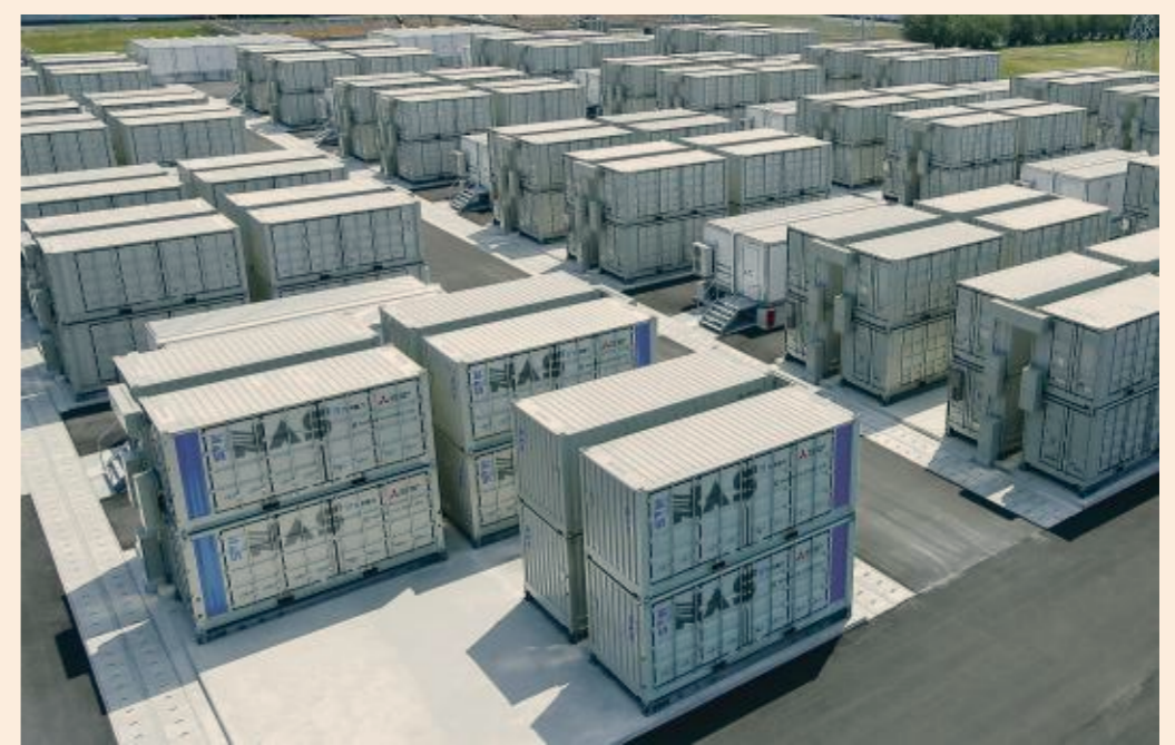
NAS systems, pictured here, are deployed at various wind and solar power stabilisation sites globally.
